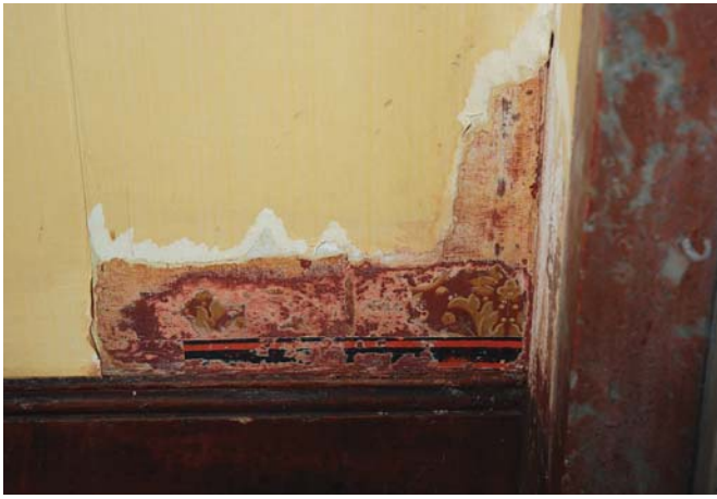
An area of the original wallpaper showing the 'black on orange' fillet border
