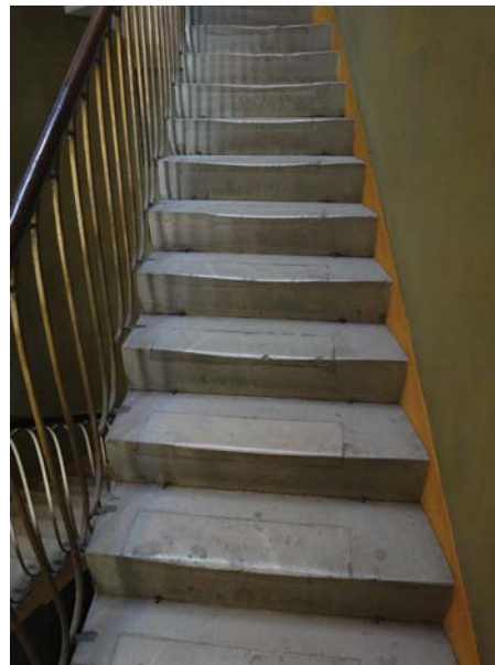
The cantilevered staircase at No.12 which will have a number of stone slabs replaced or repaired in preparation for visitors' use when the building is reopened next year. Photograph: John Bridges
