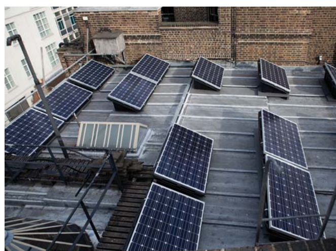
The newly installed solar panels on the roof on No.13 Lincoln's Inn Fields. Photograph: Lewis Bush
