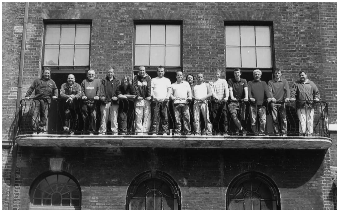
The team from Fullers Builders load test the balcony at No.14 Lincoln's Inn Fields
